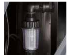
Door for inspecting and cleaning the water filter
