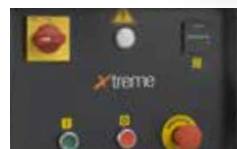
Low voltage (24V) control panel with star-delta system
