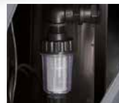
Door for inspecting and cleaning the water filter
